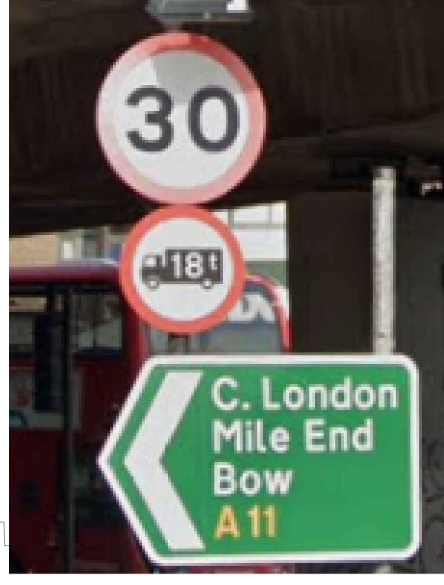
EXISTING '30MPH', DIRECTIONAL AND '18T' TRAFFIC SIGNS RELOCATED ON NEW WIDE-BASED POST.
